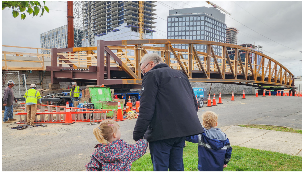
Curiosity about the construction and installation of the Wiehle overpass spans all ages of bikers, motorists, and pedestrians. Photo by Benjamin Burgess
